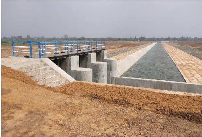
Construction of Checkdam across Pennaiyar river in Kandarakottai Village in Panruti Taluk of Cuddalore District at a cost of Rs.33 Crore.
