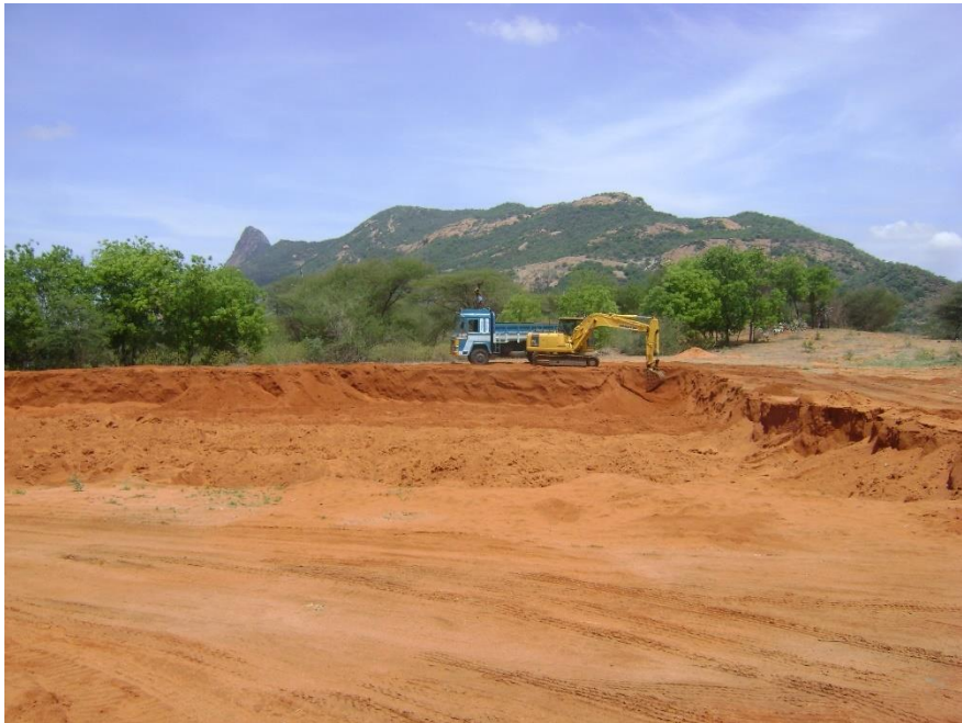
Photo: Gravel excavation at Ellapatti, Oddanchatram taluk of Dindigul District. [N10°39'12.55" E77°46'06.47"]
